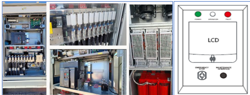
Figura 5.3: Vistas detalle componentes (HMI, Power Stack, Fusibles DC).
